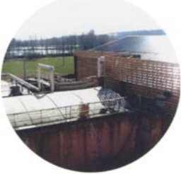
Luneville, France (2002) Simultaneous nitrification/denitrification after physical-chemical settling 4 cells, 63 m 2 each. 50 000 PE
