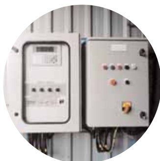
Sludge density monitoring unit.
