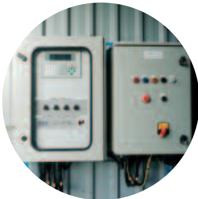
Sludge density monitoring unit
