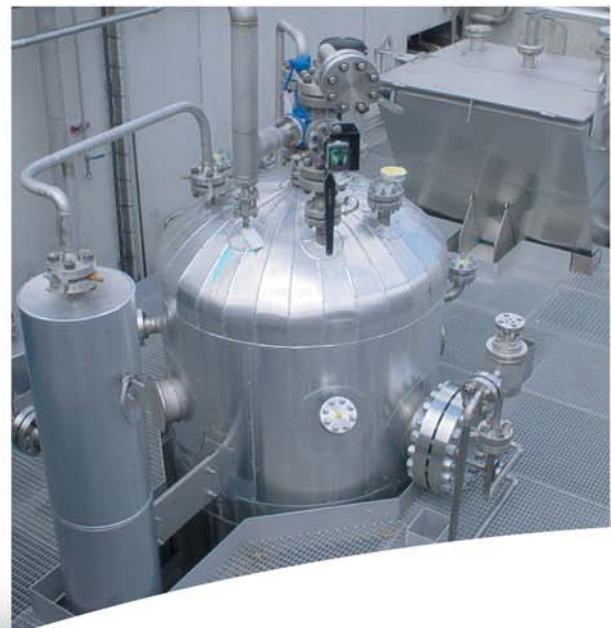
ATHOS™ unit at Epernay (France)
